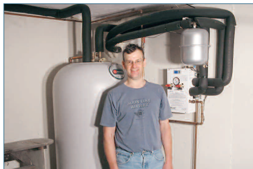
Local homeowner John Cownie had this solar hot water tank installed in his basement with Concord Light's help.
