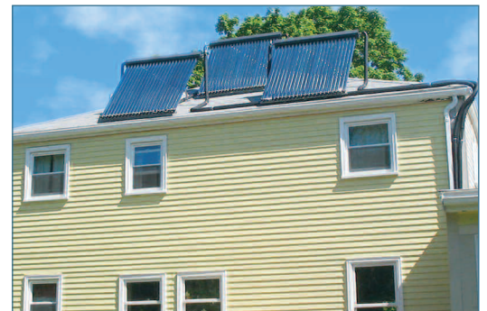
These panels on the roof of the Cownie home collect solar energy for hot water.
